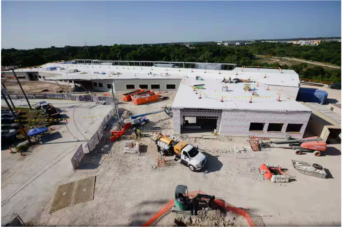
Construction continues on Metrocare's new Oak Cliff clinic in Dallas on Wednesday, July 3, 2024. The 45,000-square-foot mental health clinic will offer integrated, evidence-based care to children, adults, families, veterans, and individuals with disabilities. (Juan Figueroa / Staff Photographer)
